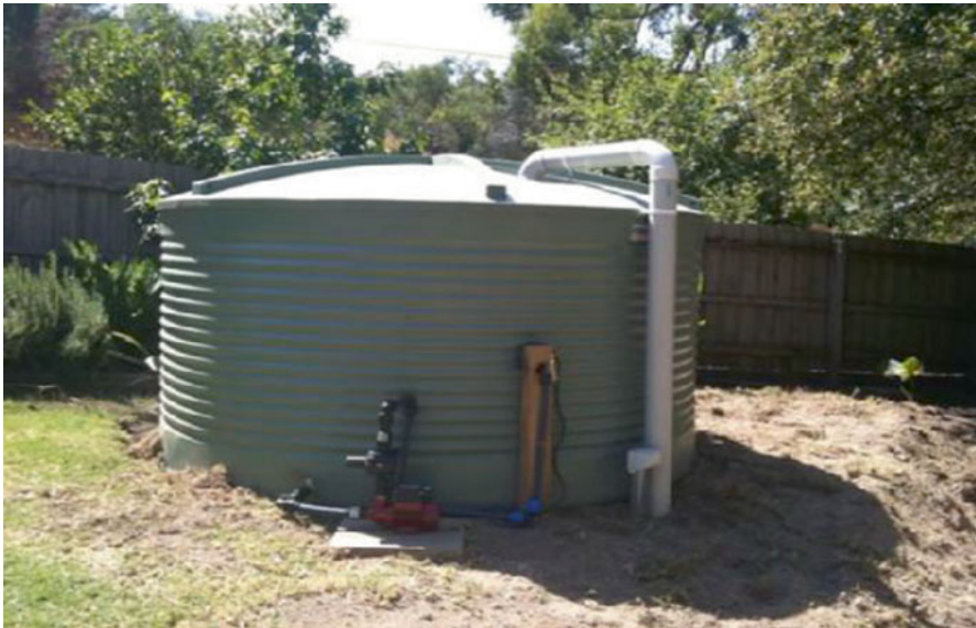
Fig. 3.2 A back yard small water storage tank
